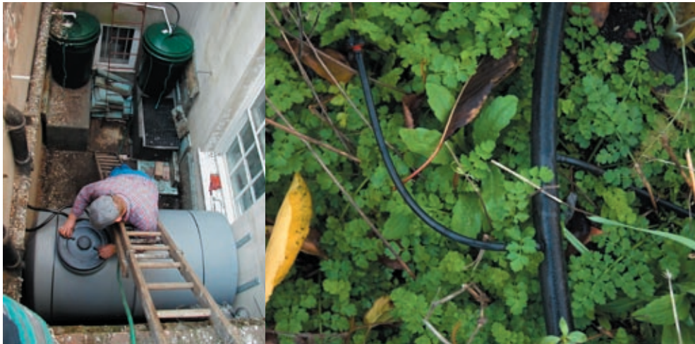
RISC's drip feed irrigation system which uses harvested rainwater
